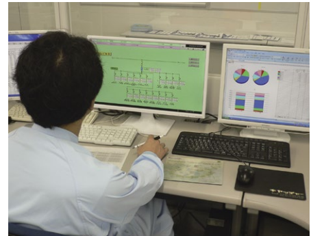
Power monitoring system of the Fukusaki Factory
